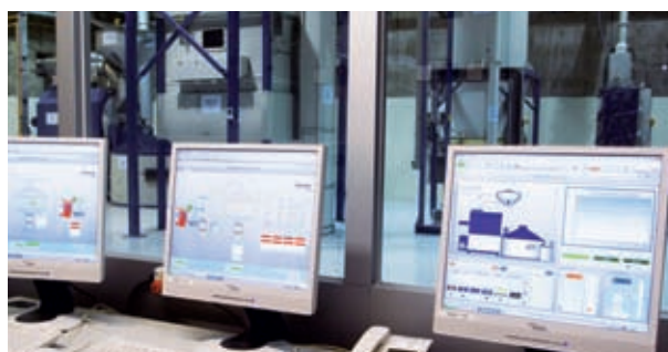
The PILOT PLANT monitors all process operations.
